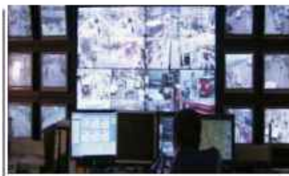
CENTRAL CONTROL ROOM
